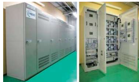
図3 伊豆大島に設置されたリチウムイオンキャパシタ設備 Figure 3 Lithium-ion capacitor systems which were installed on Izu-Oshima
