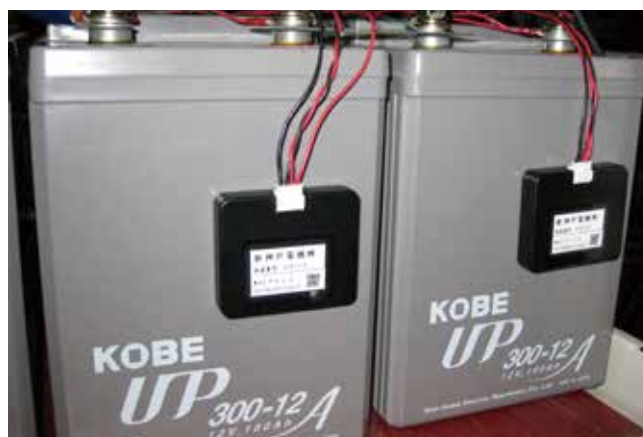
図6 無線子機を装着した試験電池の外観 Fig.6 Appearance of test battery equipped with wireless device
